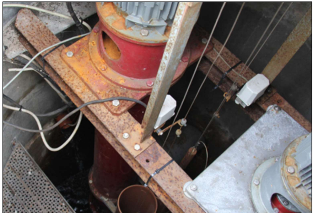
Figur 6: Pumper i pumpestationen.
